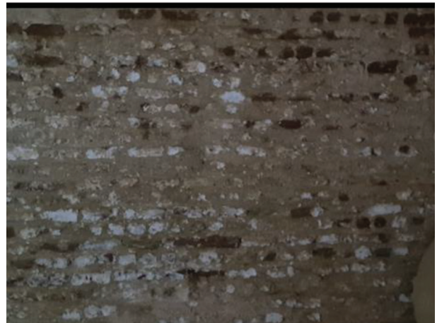
Source: Field study conducted by the researcher in July 2023. Pic. (7) The spread of salts and bacteria inside the tank in Quseir Castle.
